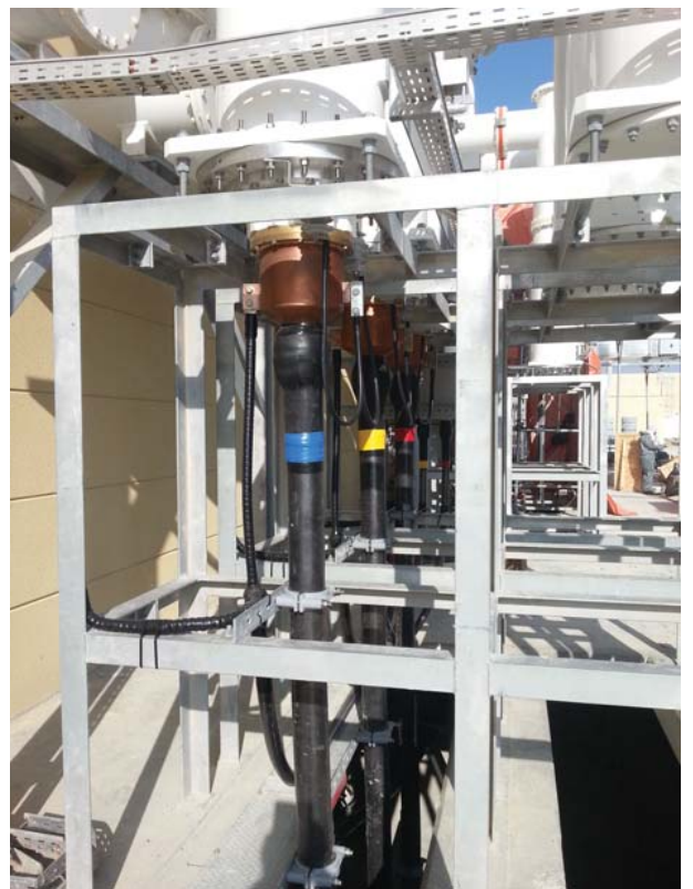
초고압 380KV, 800MM 2 XLPE Cable GIS측 종단접속 Sealing End Connection of 380KV, 800MM 2 XLPE Cable at GIS, Saudi Arabia
