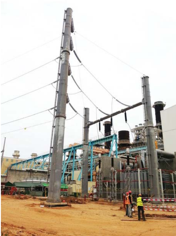
가나 T2 발전소 161KV 송전선로 인출 Drawing Out 161KV Transmission Line from Ghana T2 Power Station
