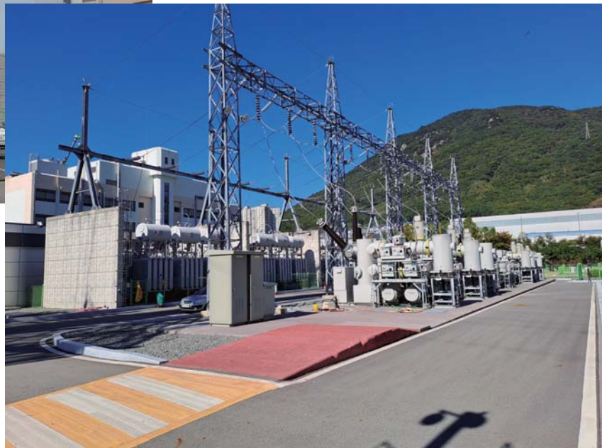
삼정변전소 옥외철구설비 GIS화 공사 GIS for Outdoor Steel Equipment at Samjeong Substation
