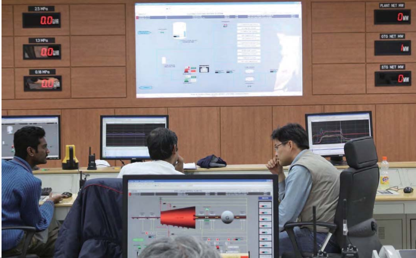
컨트롤 룸 Control Room, Armenia Yerevan CCPP
