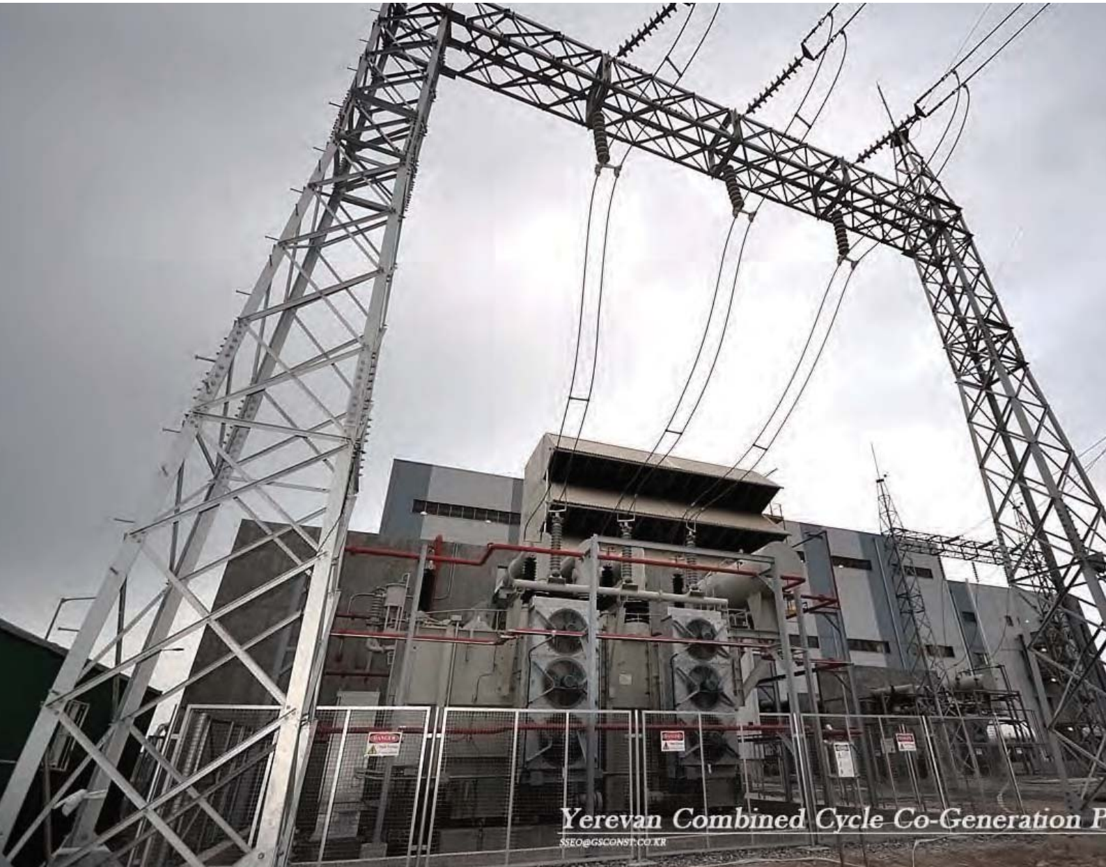
승압변압기 Step-up Transformer, Armenia Yerevan CCPP
